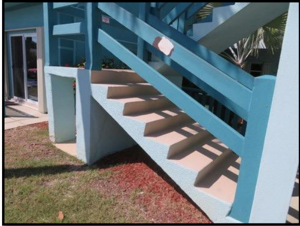
Figure 1 – Staircase Railings Spall
