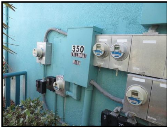
Figure 1 – Main Electric Panel
