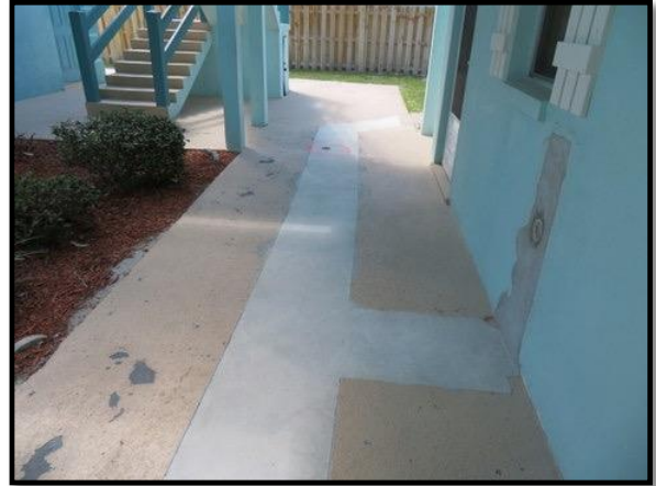
Figure 2 - Previous Repairs Building E
