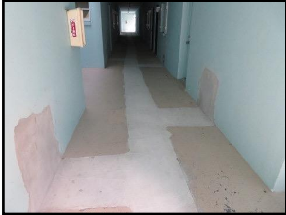
Figure 1 – Previous Repairs Building E
