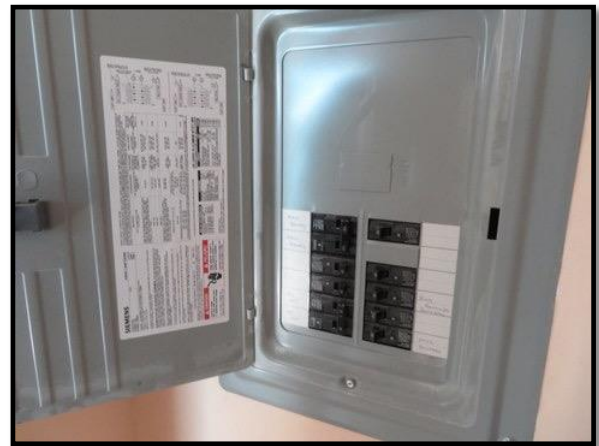
Figure 2 – Office Electric Panel
