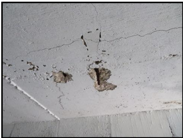
Figure 3 – Pool Equipment Spall
