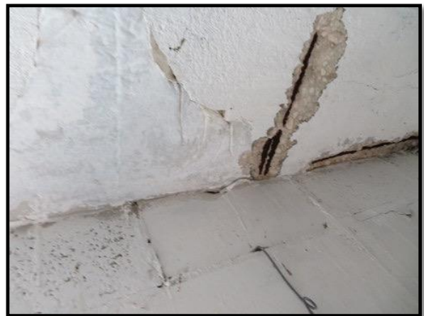
Figure 4 – Pool Equipment Spall
