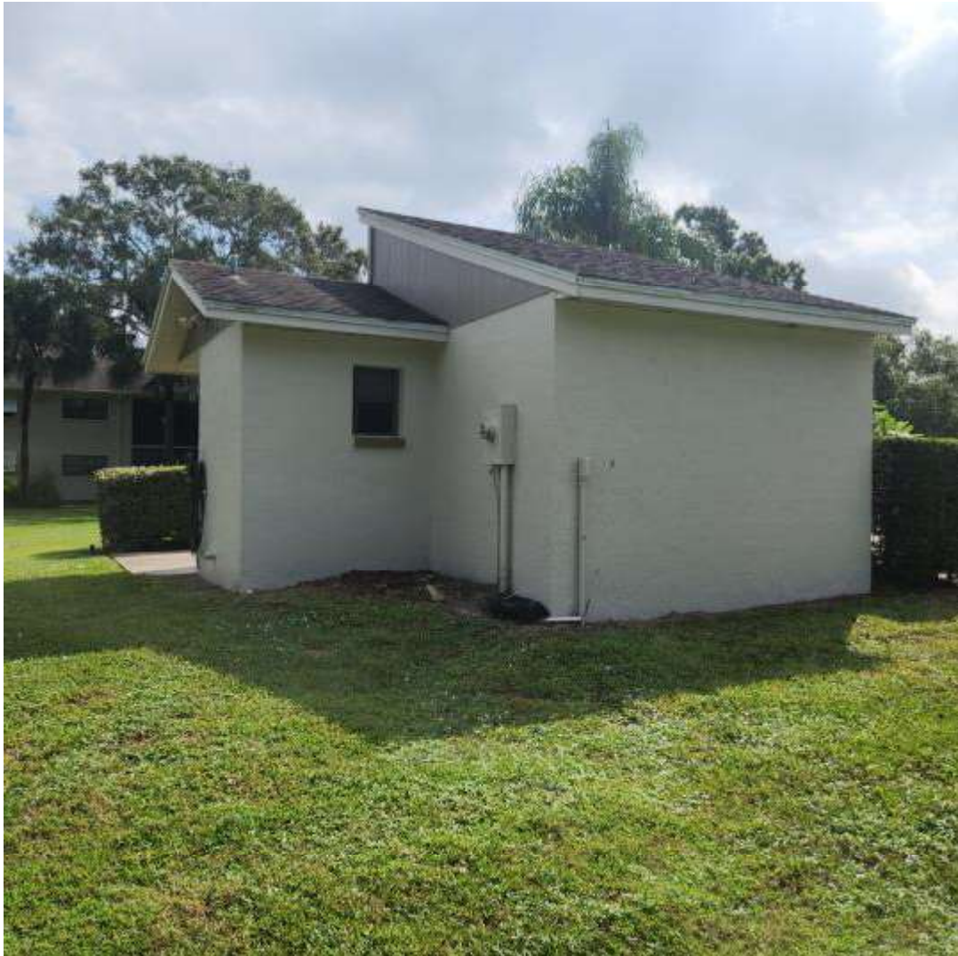
4 4-POOL RESTROOM Date Taken: 10/13/2023 Taken By: Michael Weekly THE OAKS OF COUNTRY CLUB CONDOMINIUM ASSOCIATION, INC. 1600 WOODLAND RD. ROCKLEDGE, FL 32955
