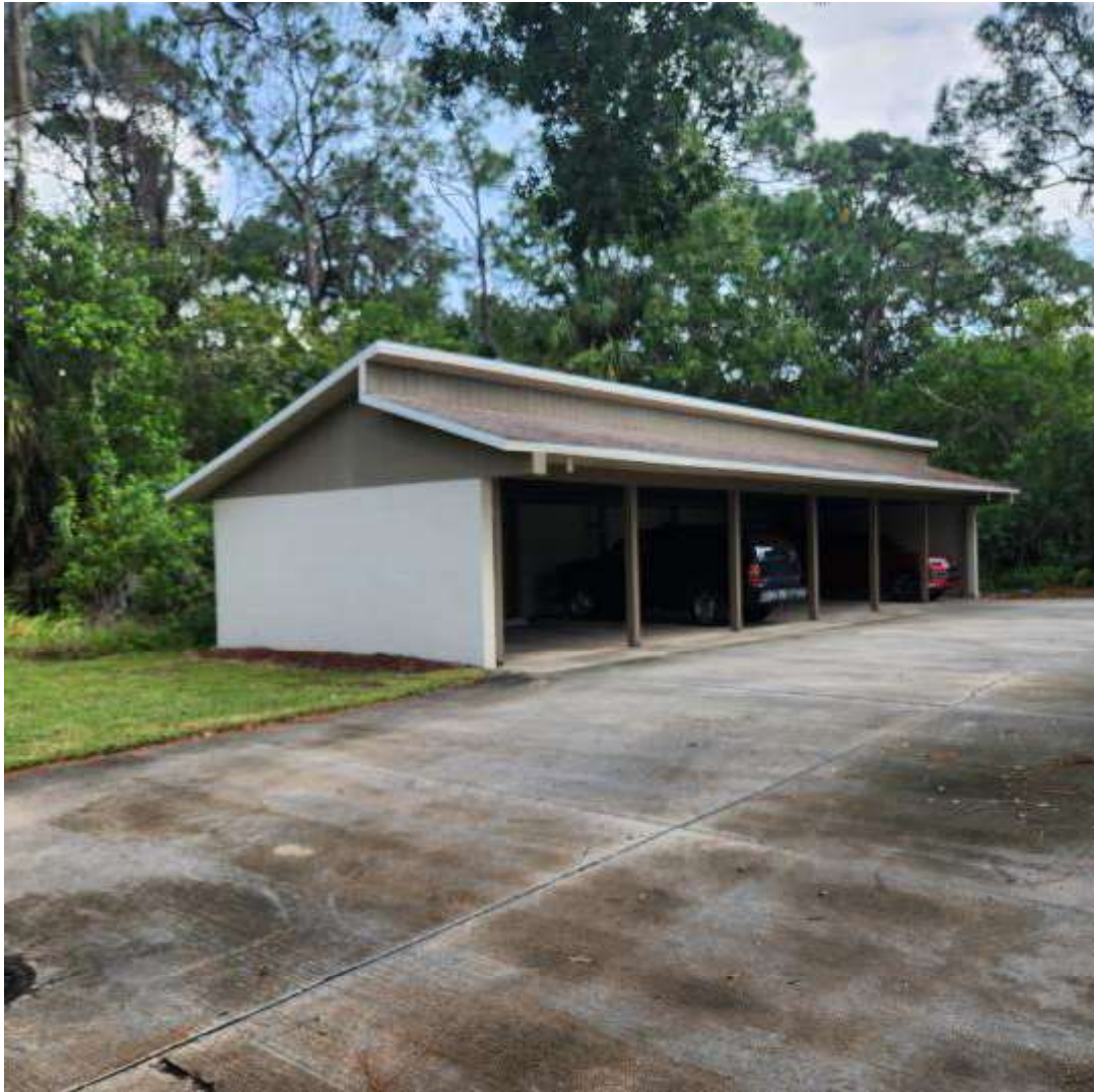
11 11-CARPORT 1 Date Taken: 10/13/2023 Taken By: Michael Weekly THE OAKS OF COUNTRY CLUB CONDOMINIUM ASSOCIATION, INC. 1600 WOODLAND RD. ROCKLEDGE, FL 32955
