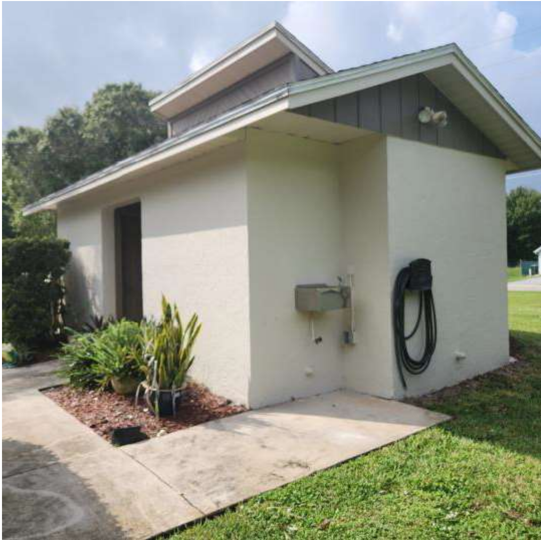
3 3-POOL RESTROOM Date Taken: 10/13/2023 Taken By: Michael Weekly THE OAKS OF COUNTRY CLUB CONDOMINIUM ASSOCIATION, INC. 1600 WOODLAND RD. ROCKLEDGE, FL 32955
