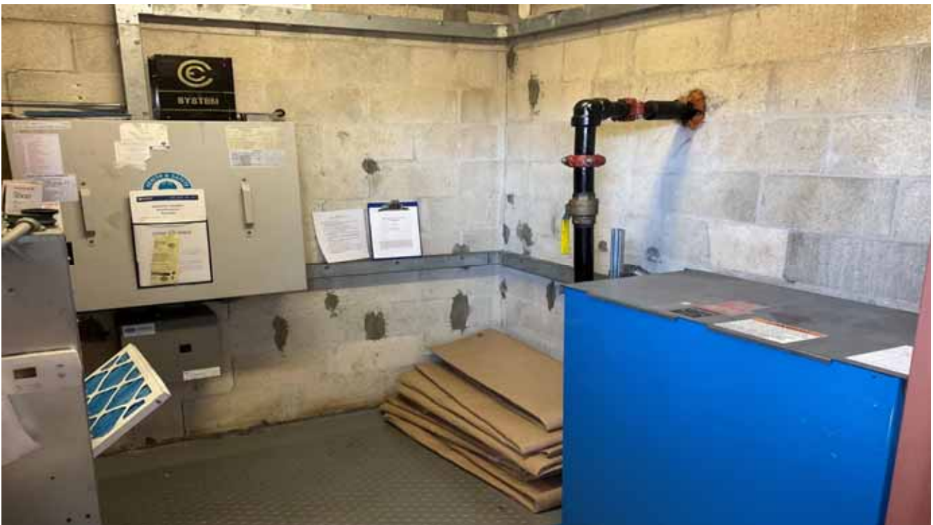
2300 Bldg - Elevator Equipment
