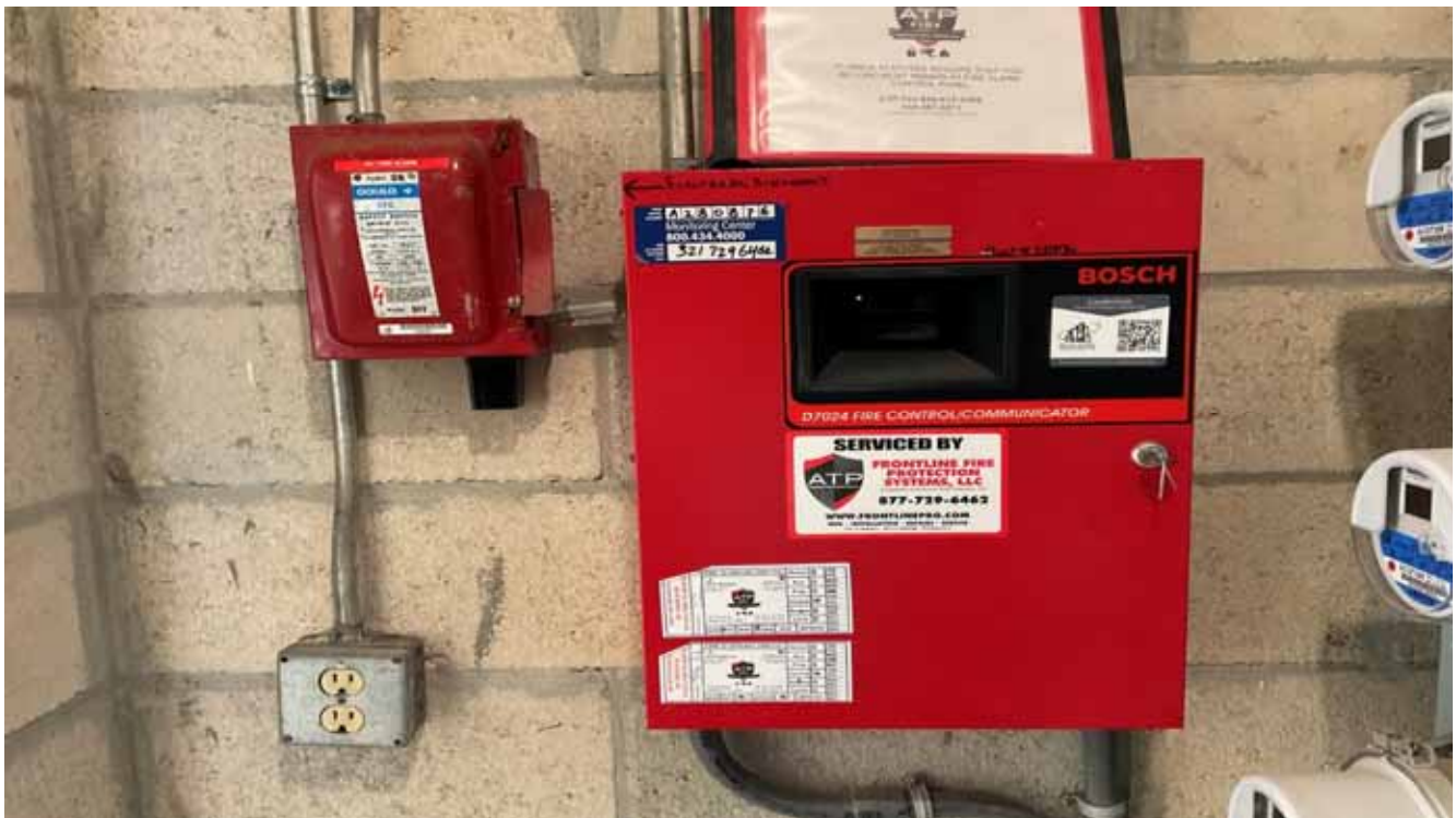
2400 Bldg - Fire Alarm Panel
