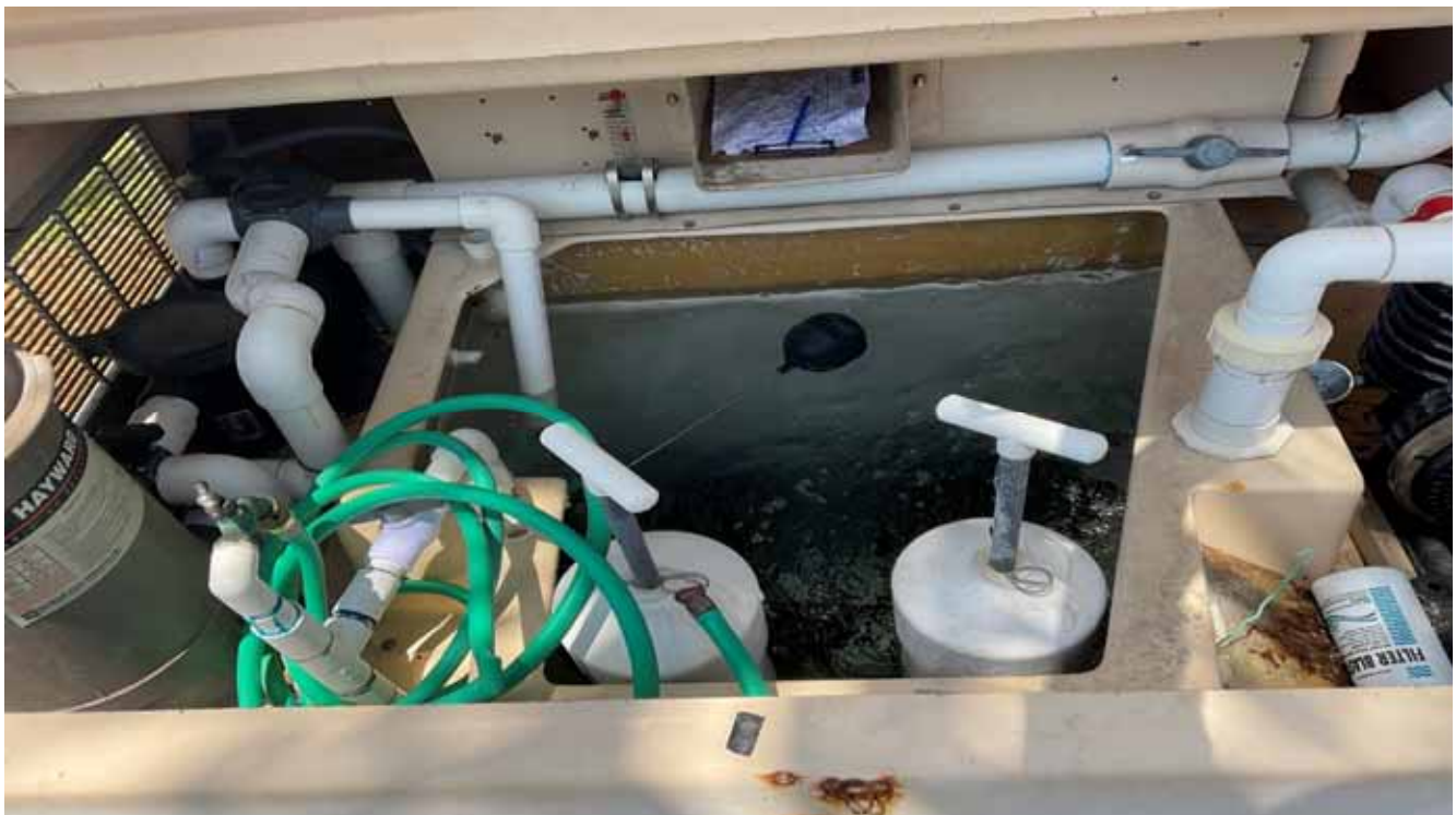
Pool Equipment - Midrise
