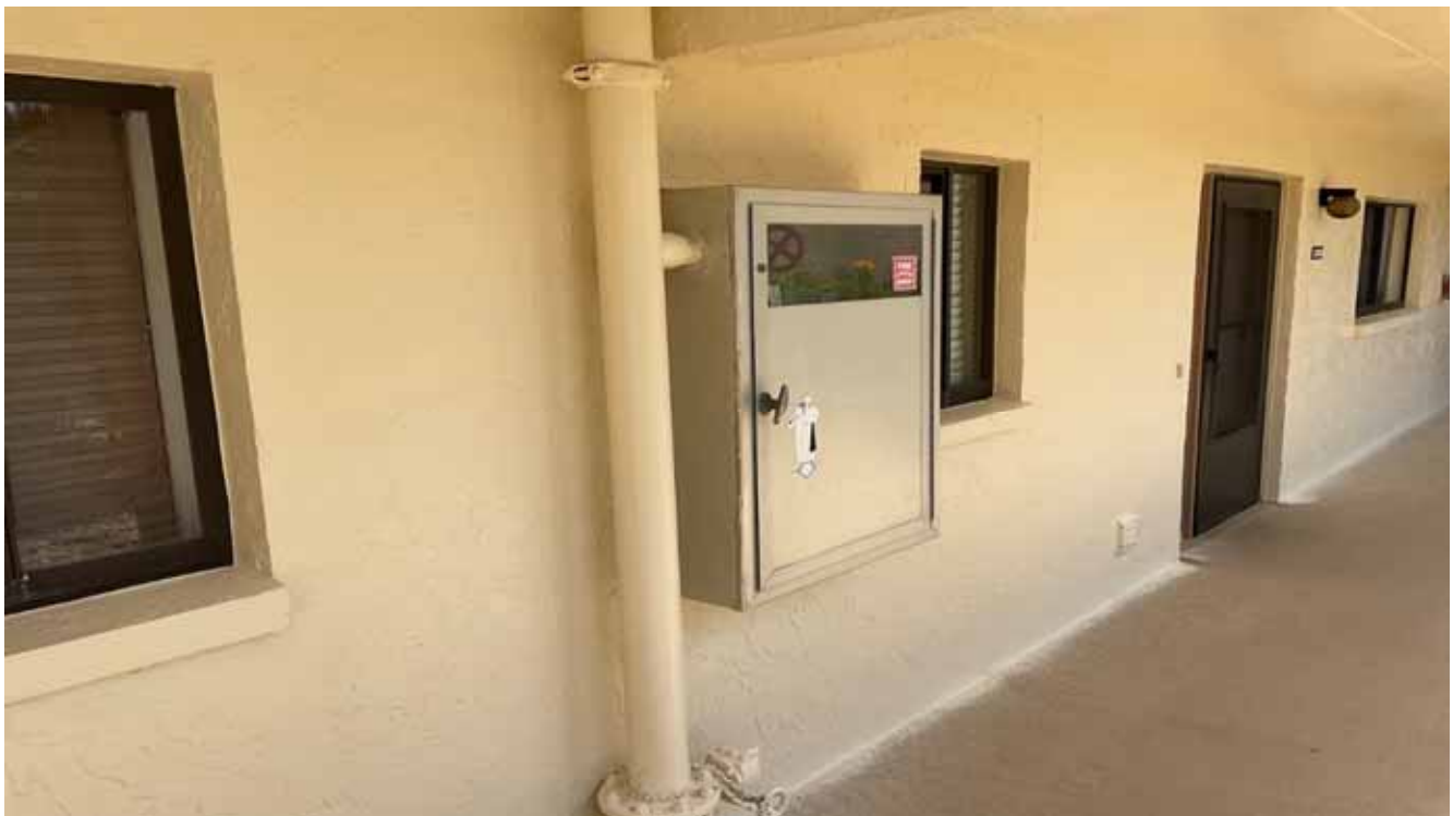
Fire Standpipe Riser
