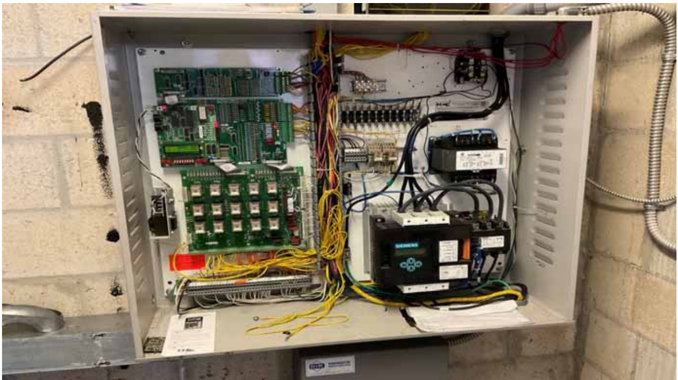
2400 Bldg - Elevator Equipment
