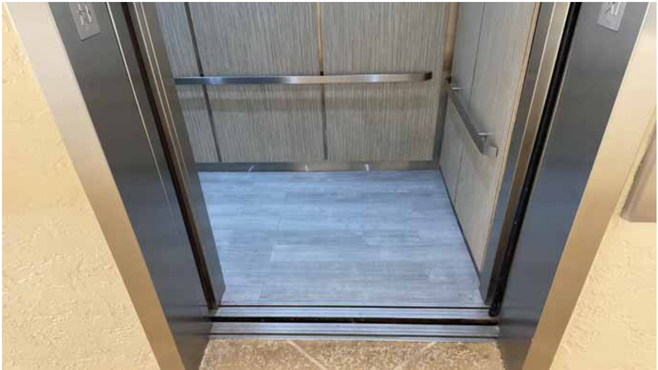
2300 Bldg - Elevator Cab
