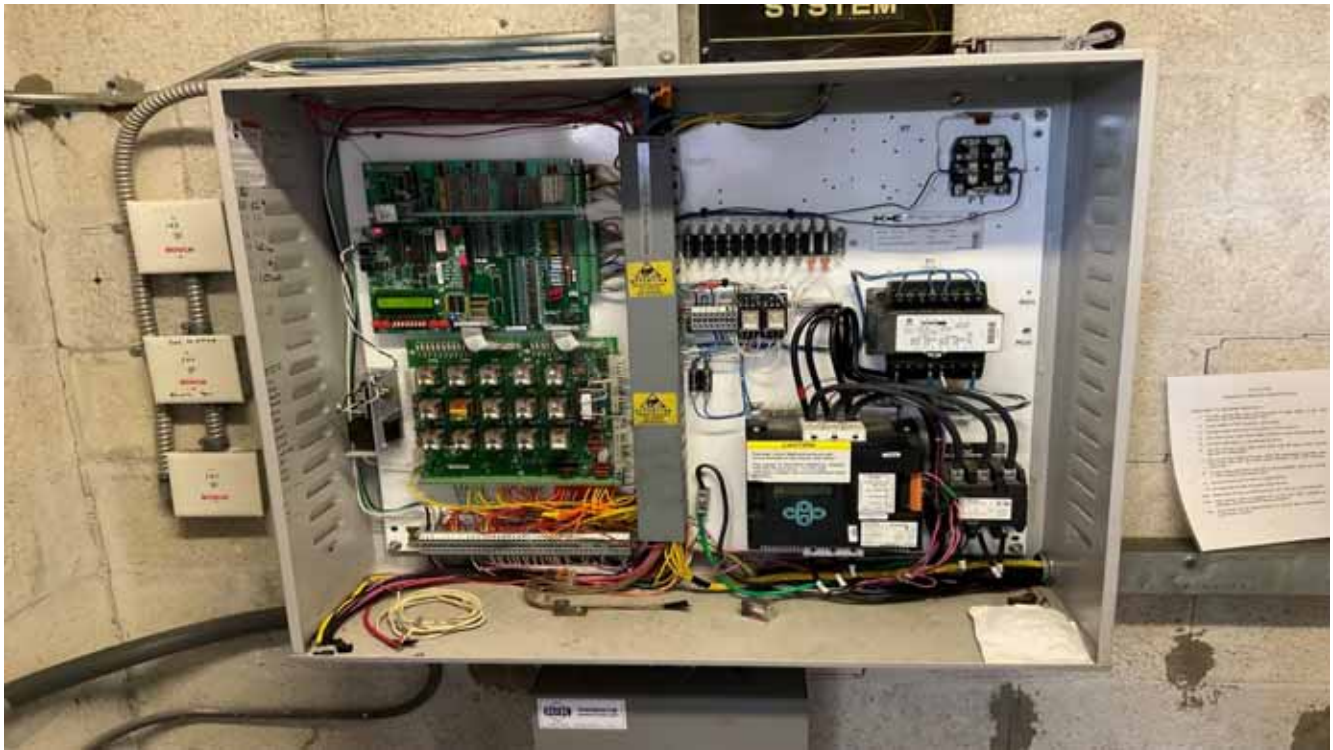
2300 Bldg - Elevator Equipment
