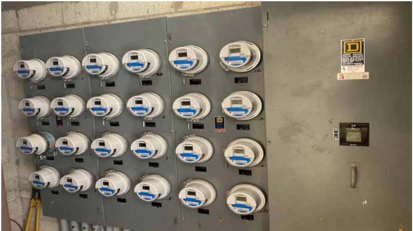
2300 Bldg - Electrical Meters
