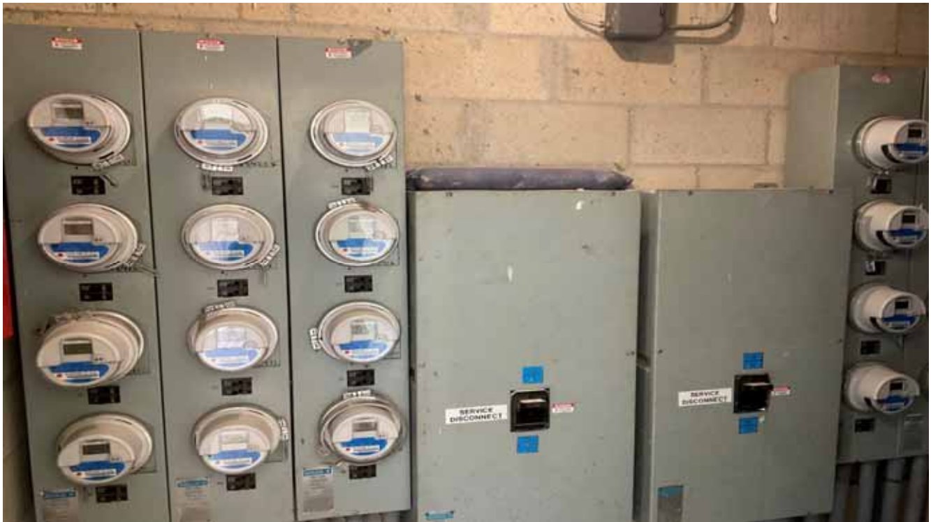
2400 Bldg - Electrical Meters
