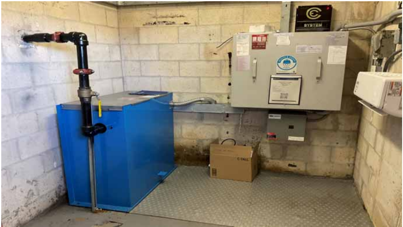
2400 Bldg - Elevator Equipment
