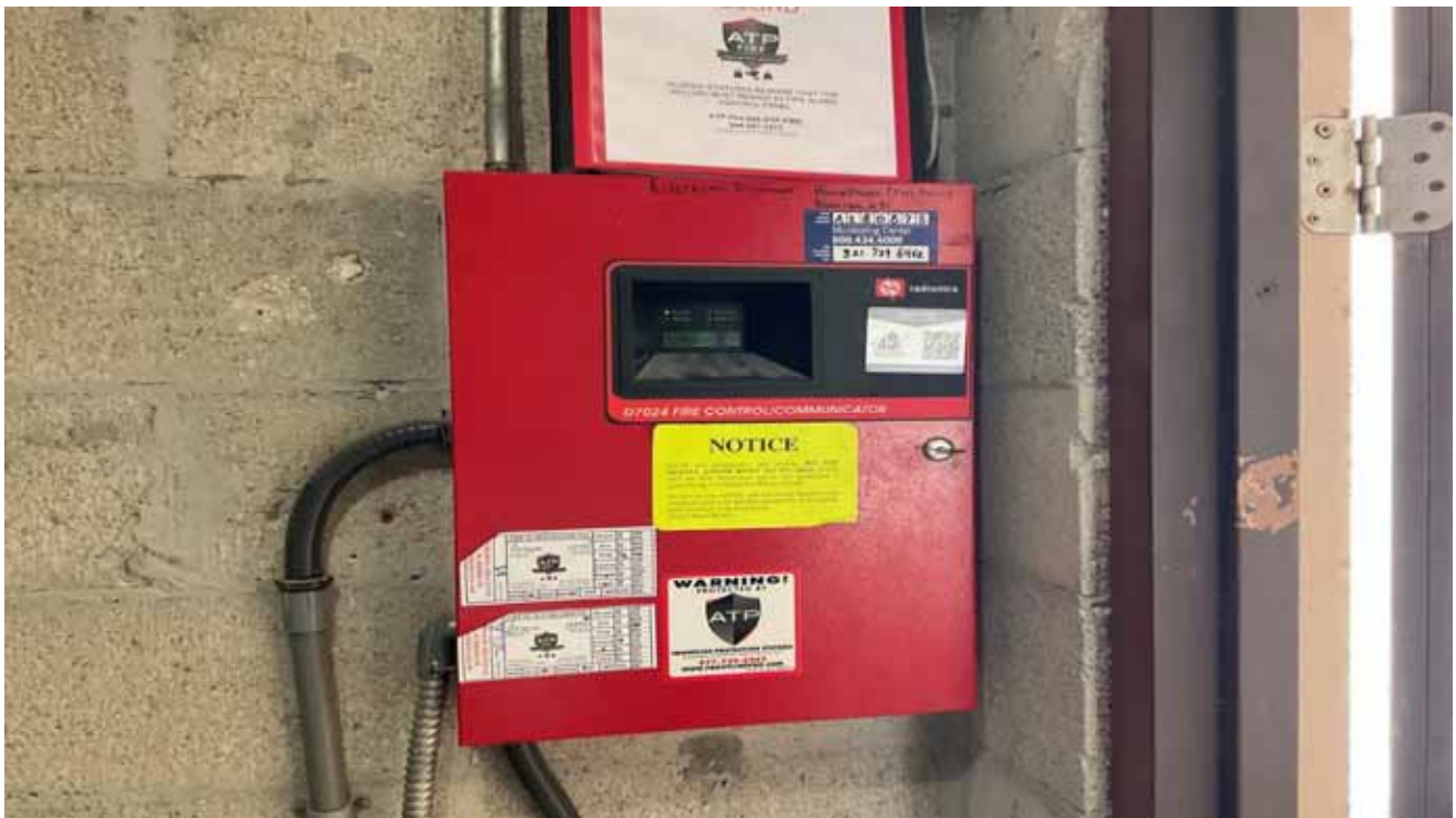
2300 Bldg - Fire Alarm Panel
