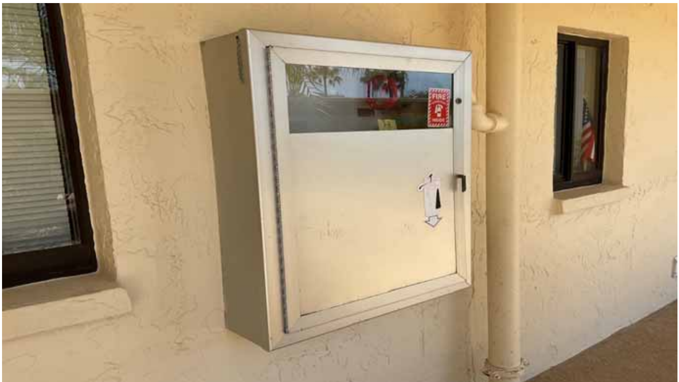
Fire Standpipe Riser
