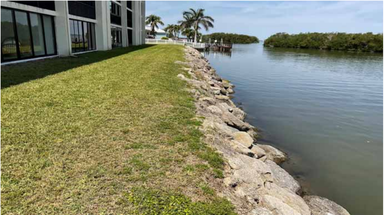
Rip Rip at Waterline
