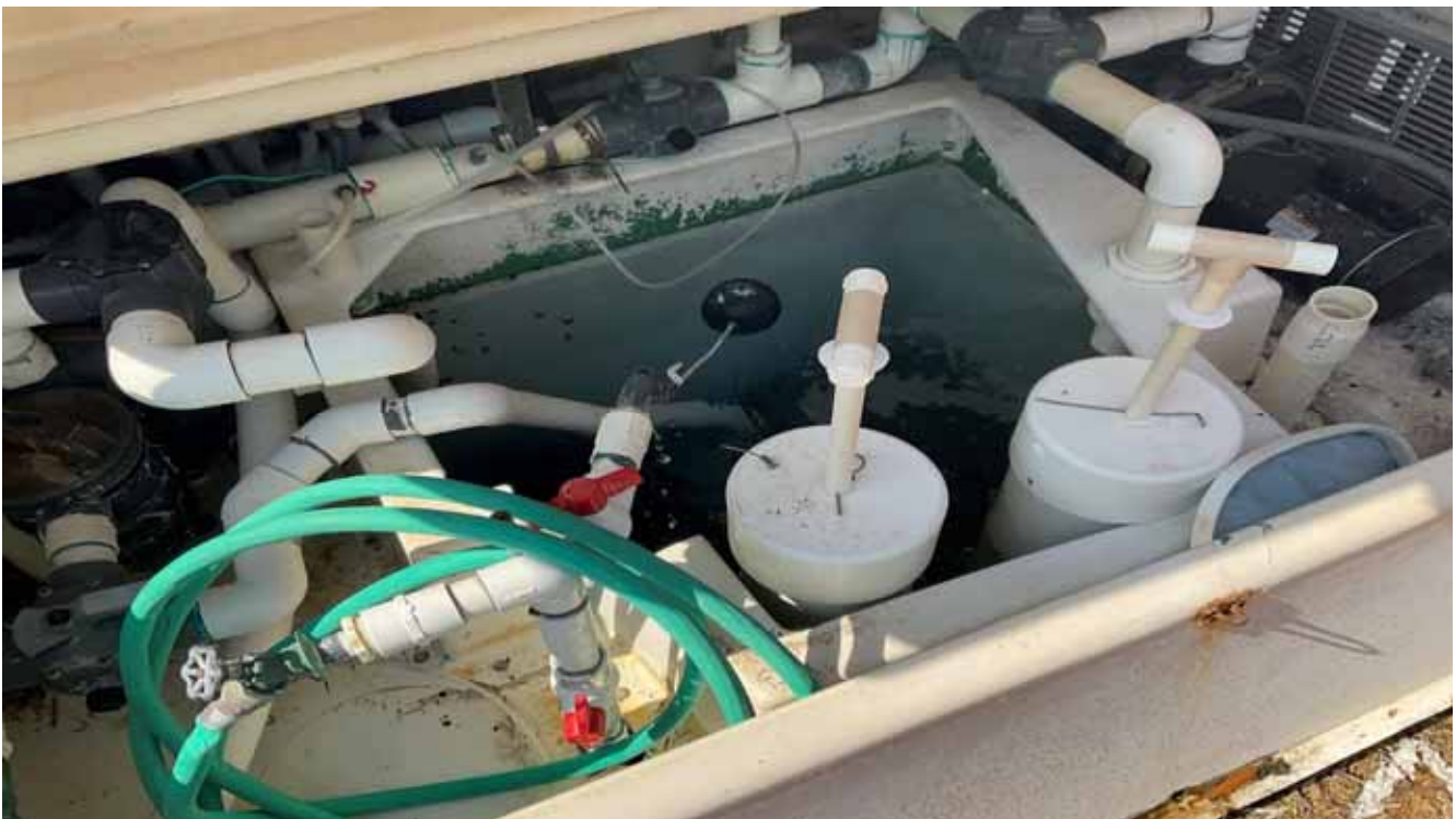
Pool Equipment - Clubhouse
