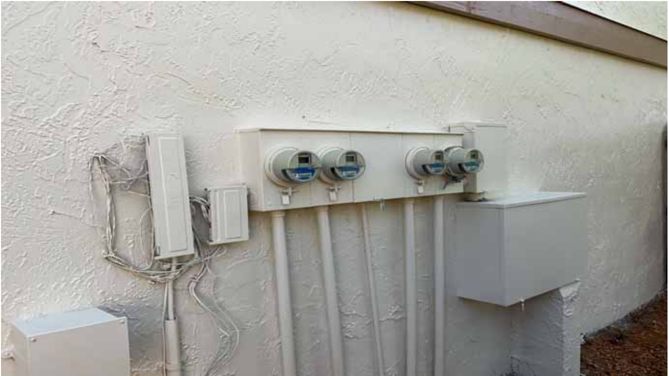
Electrical Meters at Villas - Typical
