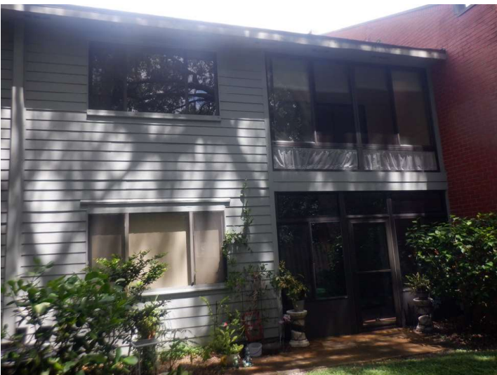
Openings not protected
