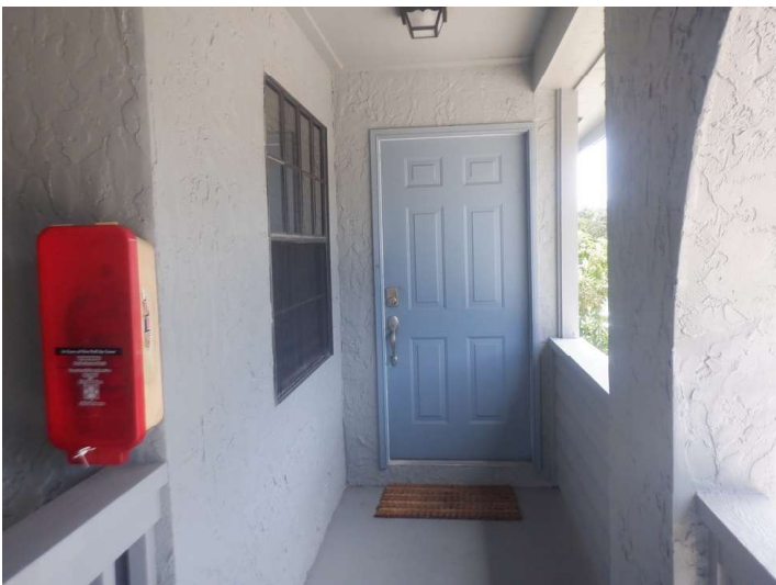
Openings not protected
