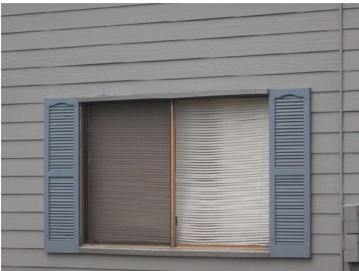
Openings not protected
