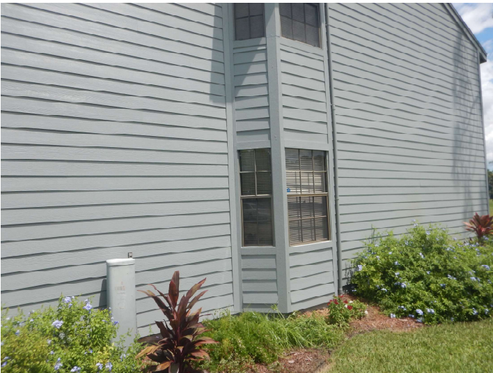
Openings not protected
