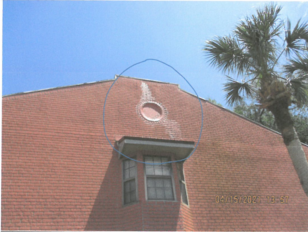
Building 1795-Example photo of brick façade stucco damage
