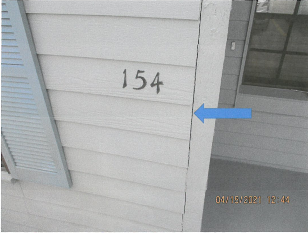
Building 1685-Example photo of needed sealant at siding transition
