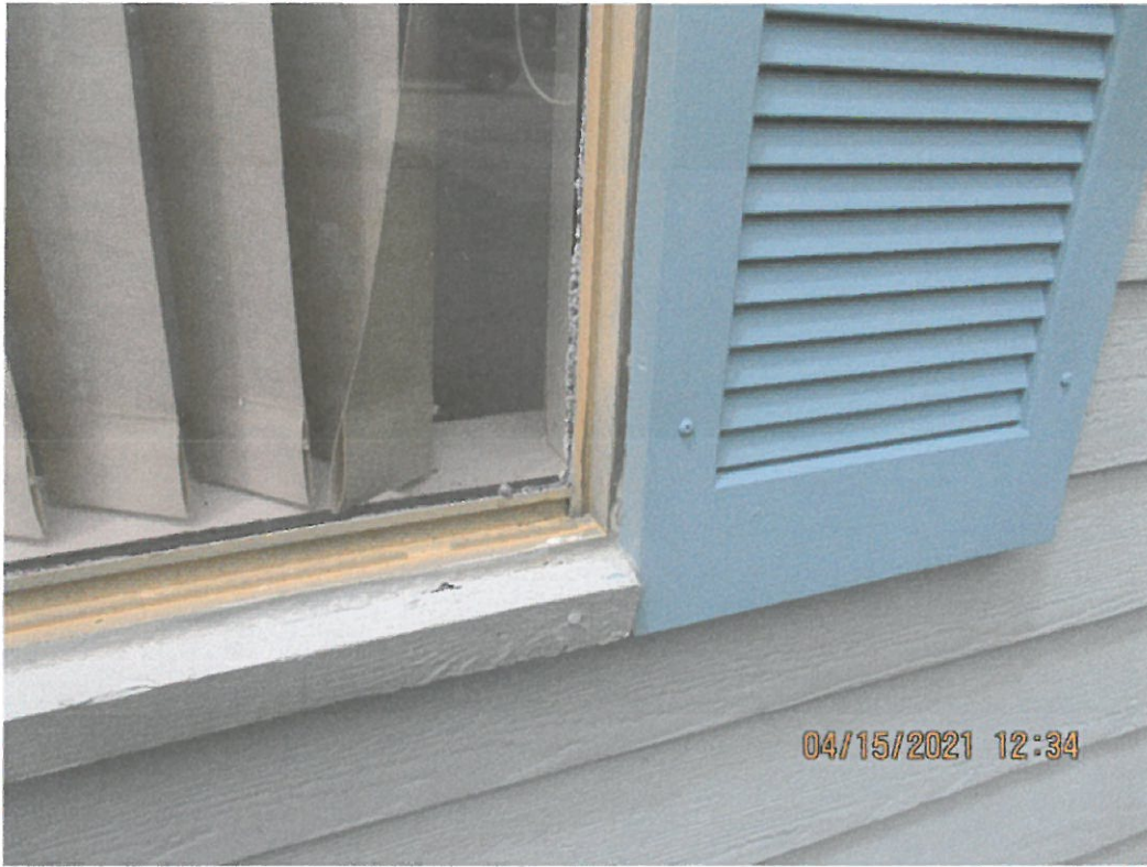
Building 1685-Example photo of aged windows-owners should consider replacement/upgrade
