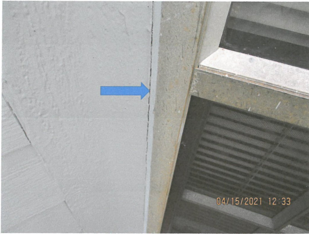
Building 1685-Example photo of needed window perimeter sealant
