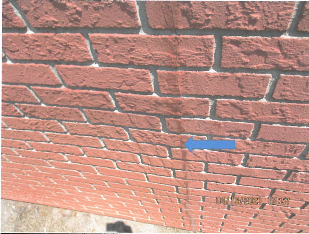
Building 1795-Example photo of brick façade stucco cracking
