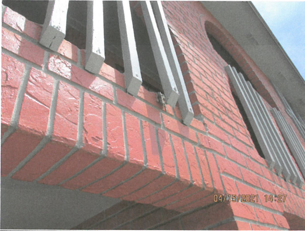
Building 1745-Example photo of loose walkway railings-advised management to have repaired during inspection process
