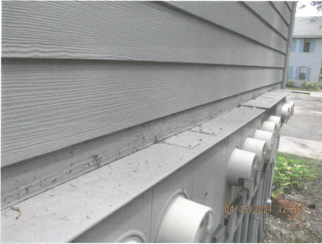
Building 1705-Example photo of sealant needed at electrical meter to wall intersection
