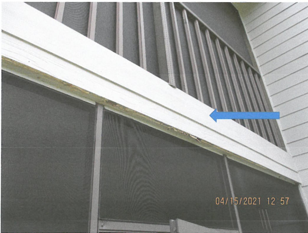
Building 1705-Example photo of rotted wood due to blocked balcony drainage from above
