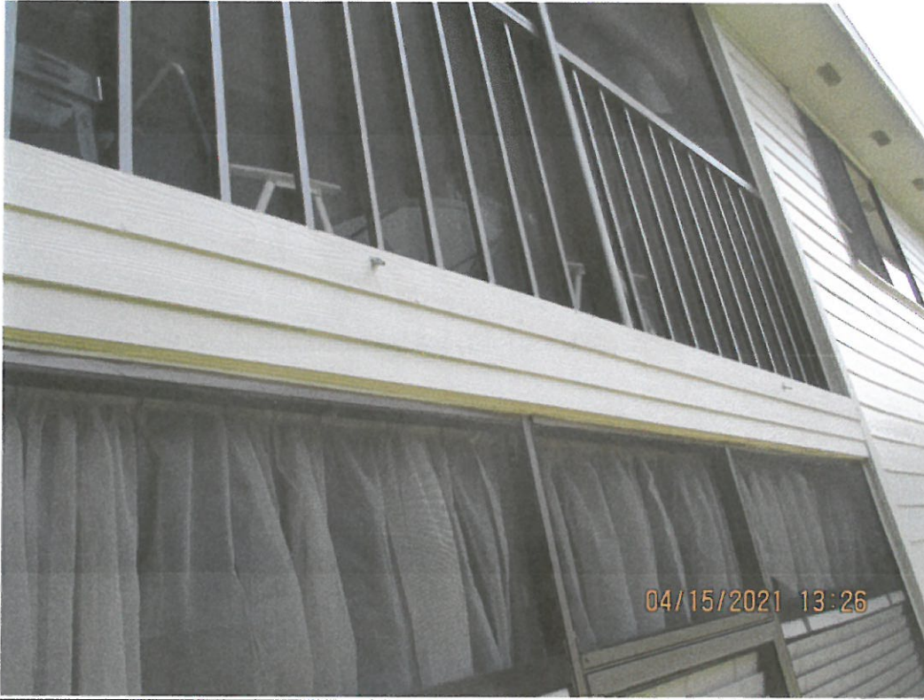
Building 1715-Example photo of added drain outlets in an ineffective attempt to create balcony drainage
