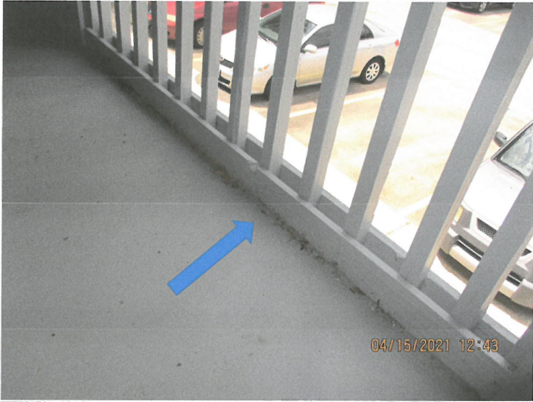
Building 1685-Example photo of blocked drainage on walkway-need to raise bottom horizontal rail
