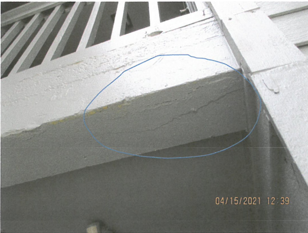
Building 1685-Example photo of concrete spall needing repaired before painting
