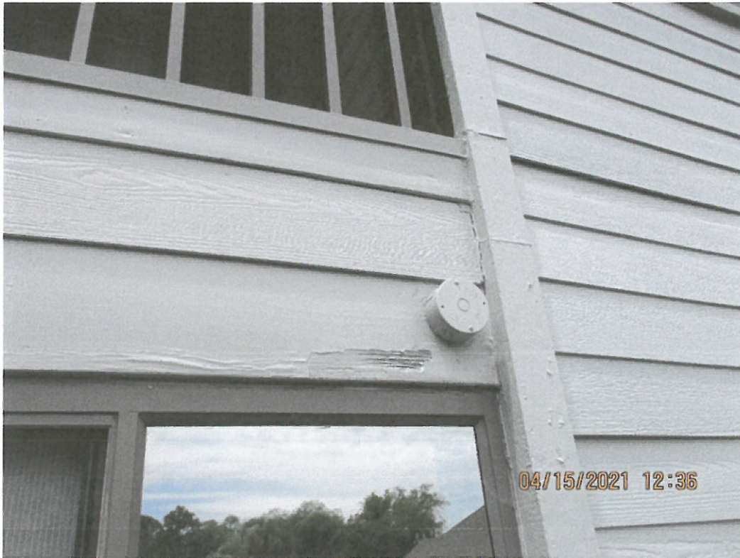
Building 1685-Example photo of rotted wood for repair before painting-probable drainage issue from balcony above
