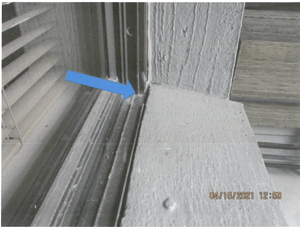
Building 1705-Example photo of wood sill blocking window weep drainage that should be repaired before painting
