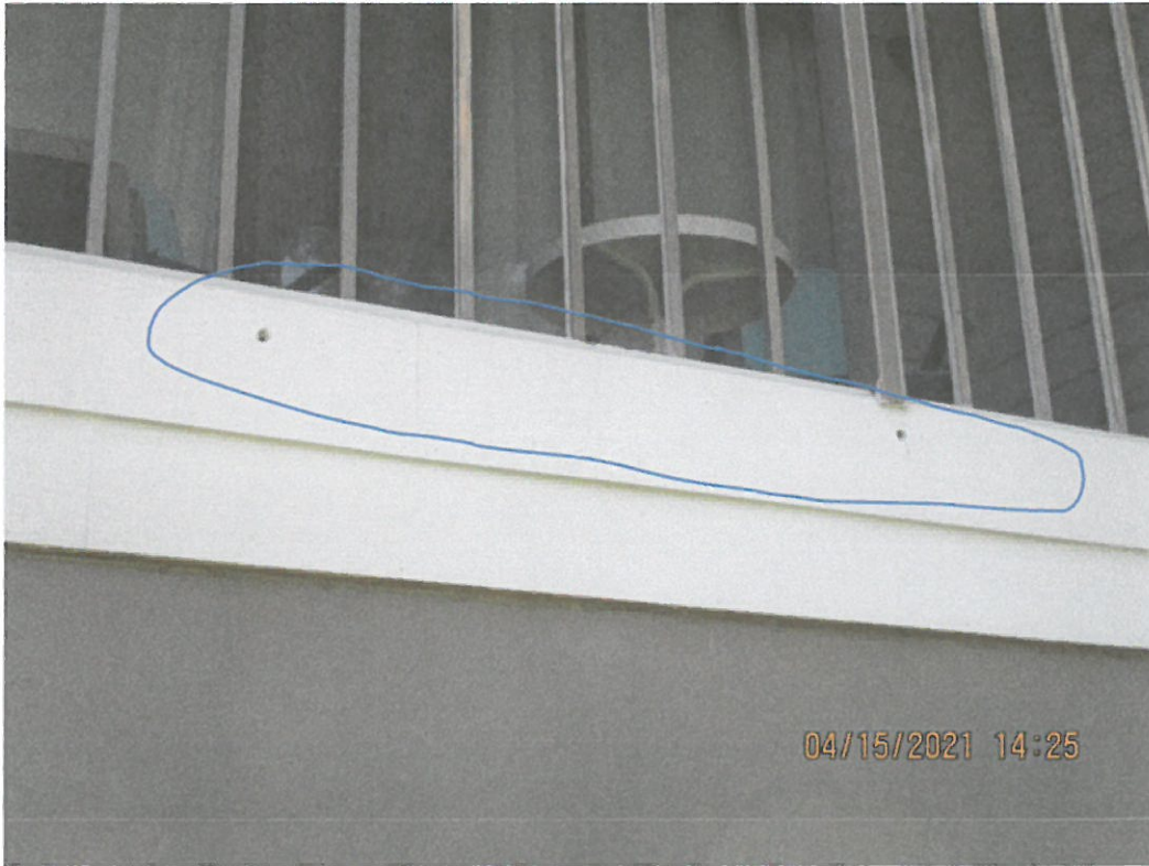
Building 1745-Example photo of blocked balcony drainage
