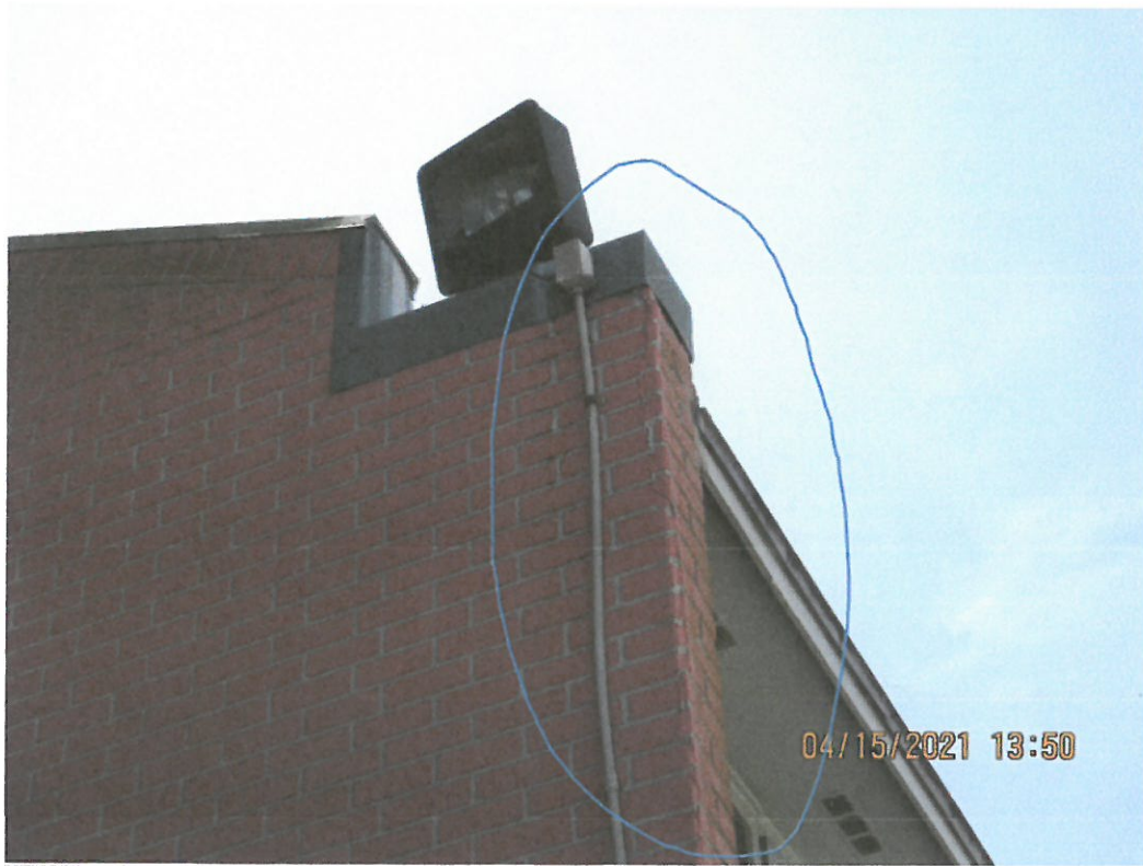
Building 1795-Example photo of brick façade column stucco/spall damage
