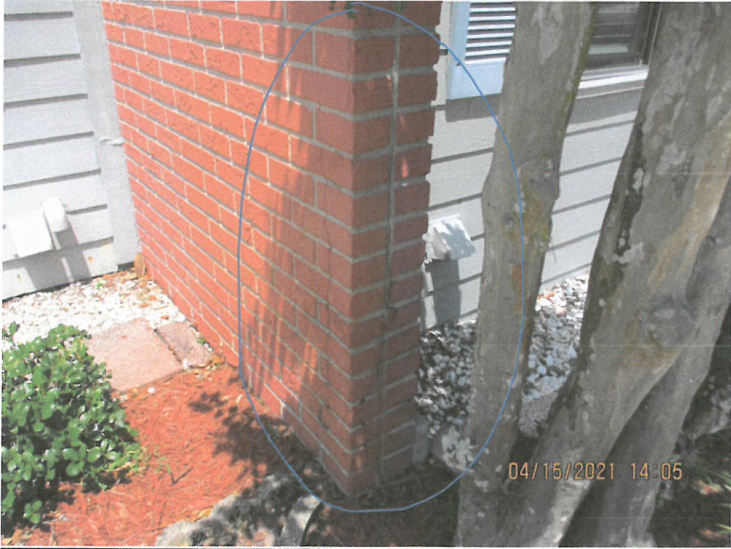
Building 1785-Example photo of cracking/spalling of brick façade stucco
