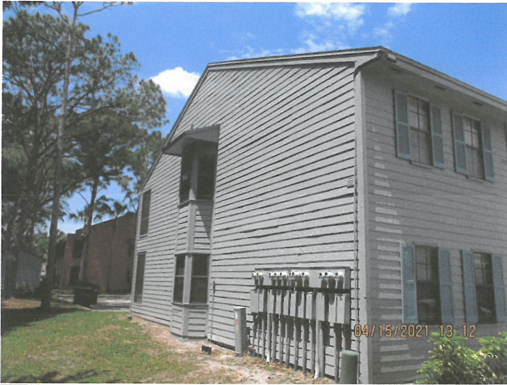
Building 1755-Example photo of wavy, warped siding likely due to improper fastening
