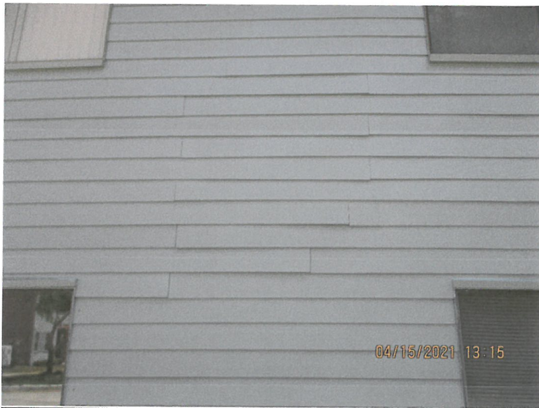
Building 1755-Example photo of poorly staggered siding laps
