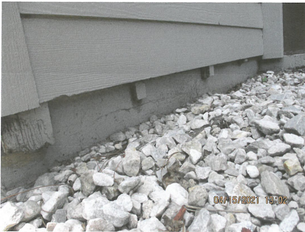
Building 1735-Example photo of siding attached to block walls with vertical wood furring strips
