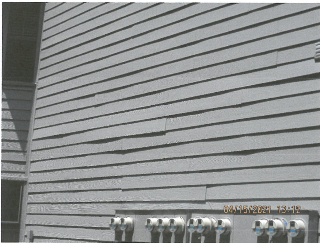
Building 1755-Example photo of wavy, warped siding likely due to improper fastening
