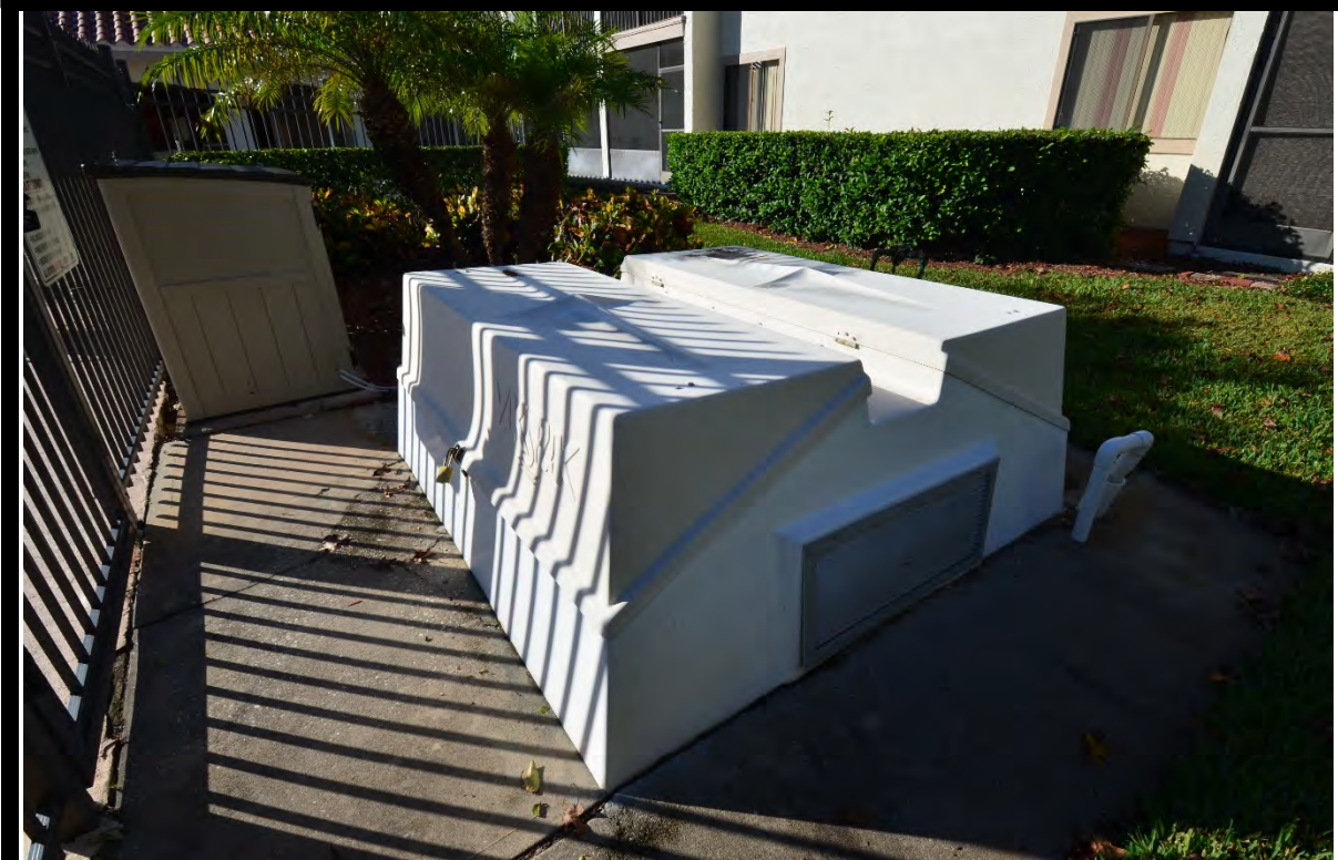
VIEW OF TYPICAL POOL EQUIPMENT
