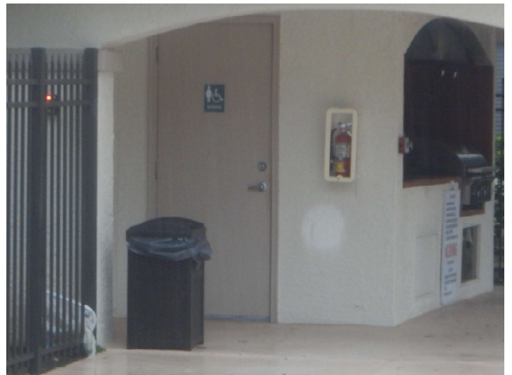
Non glazed openings not protected
