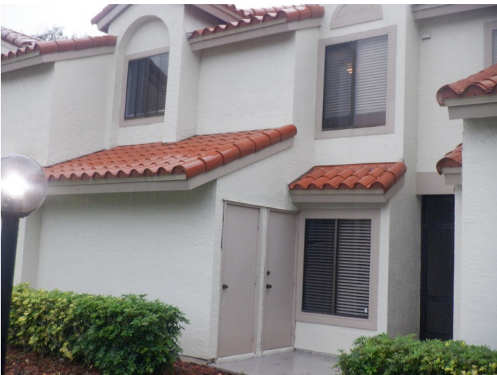
No openings protected
