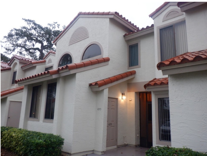
No openings protected
