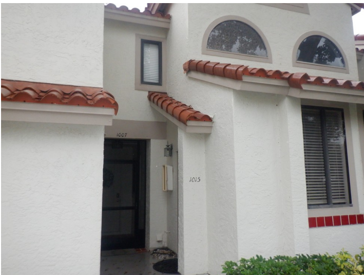
No openings protected
